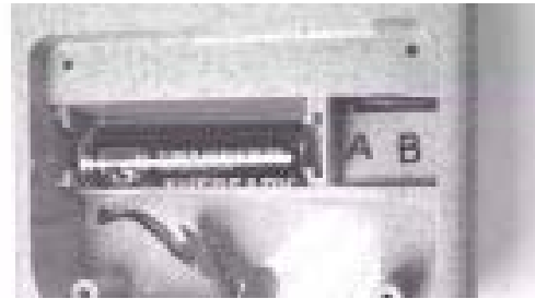
9V alkaline battery Back up power
